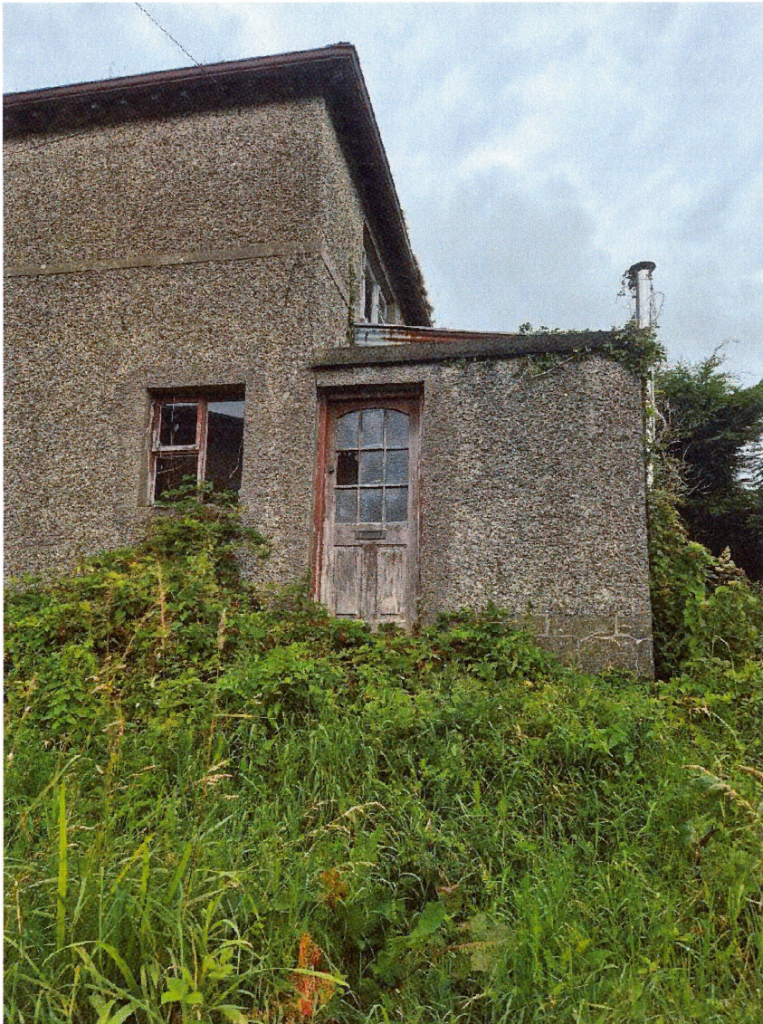
Photo 5 Rear extension and broken window panels
